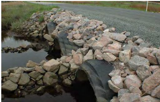
Figure 14: Roadway Drainage Crossing in the Southeastern Portion of the County.
